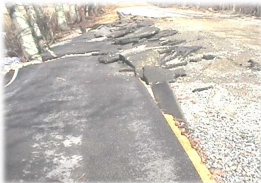
Road Damage during flood event Photo Credit: Bob Belmore, City of Somersworth
