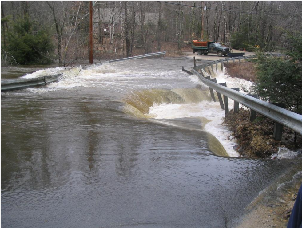
Al Fernald Bridge on McCrillis Road, April 2007 Flooding Event
