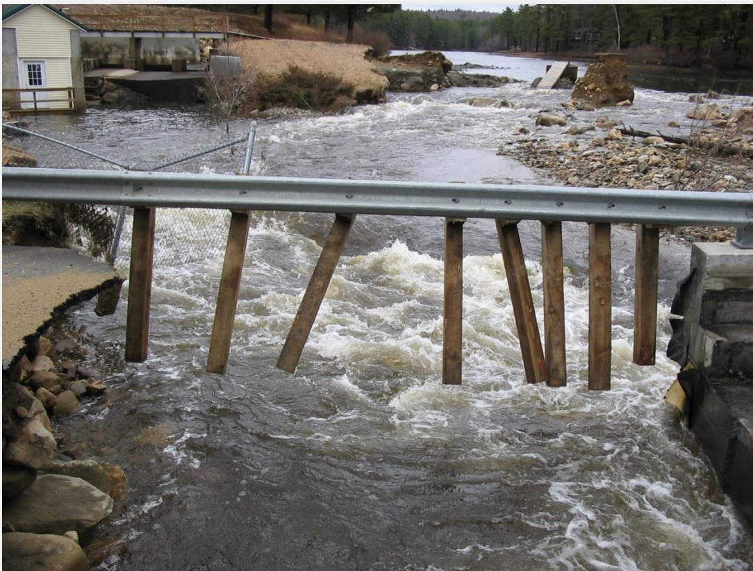
Mill Pond Bridge, April 2007 Flooding Event
