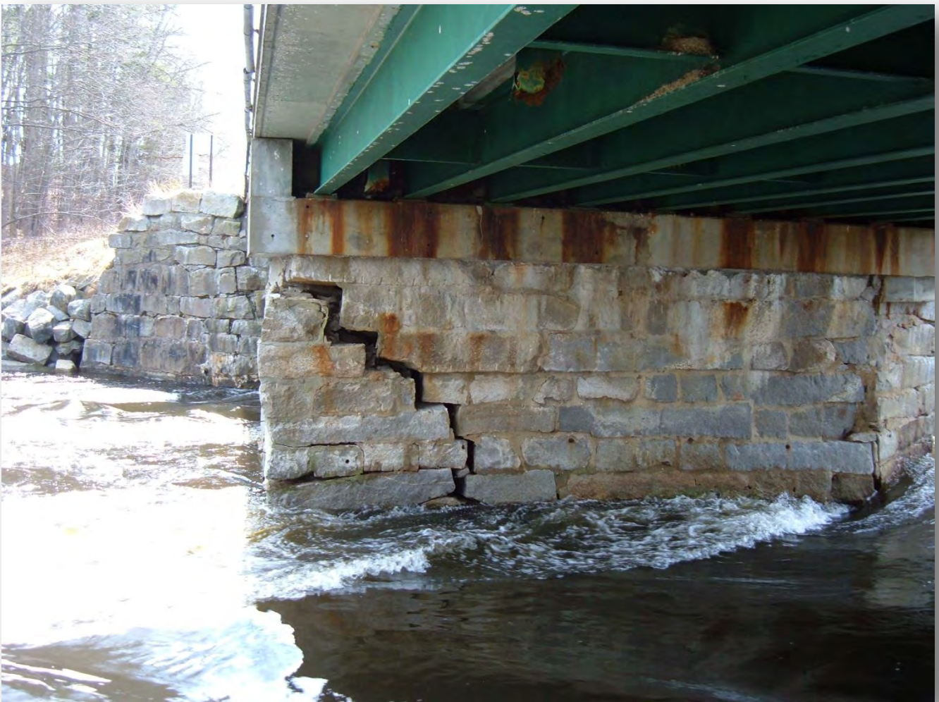
Damage to Lee Hook Road, Flooding
