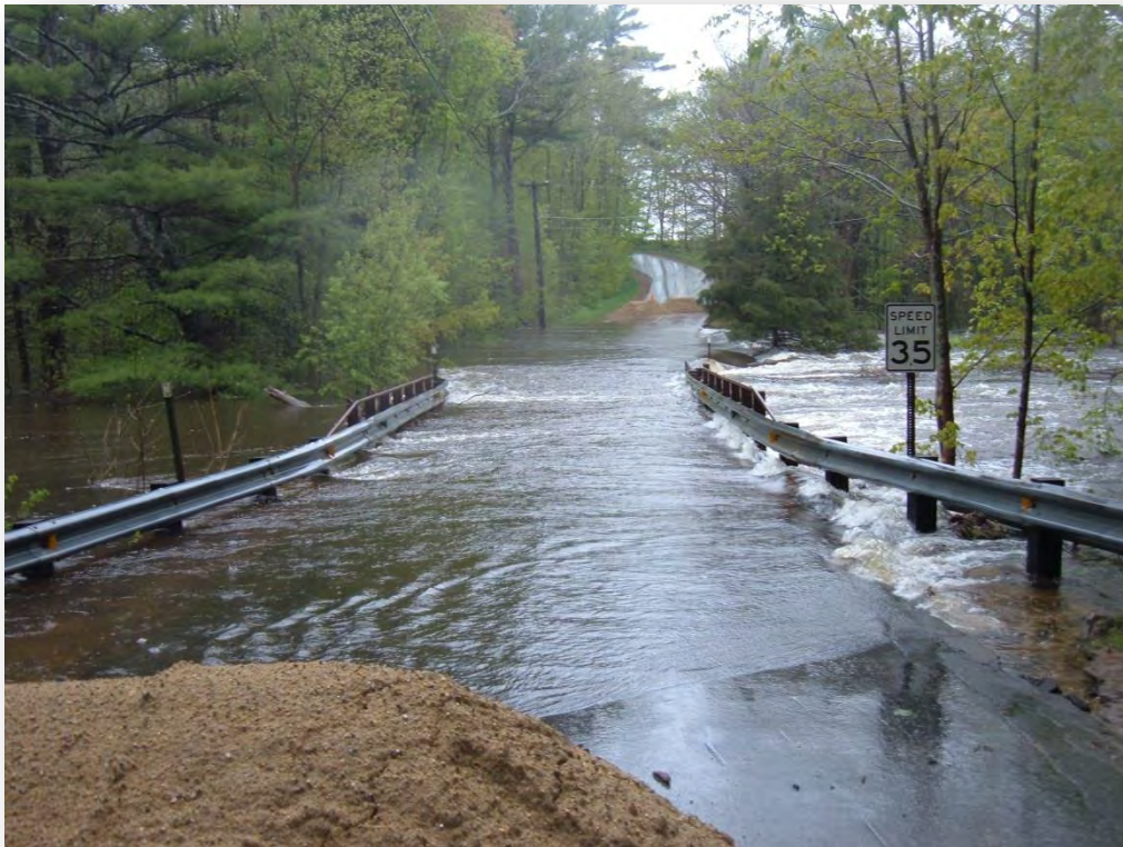
High Road Bridge, May 2006 Flooding Event
