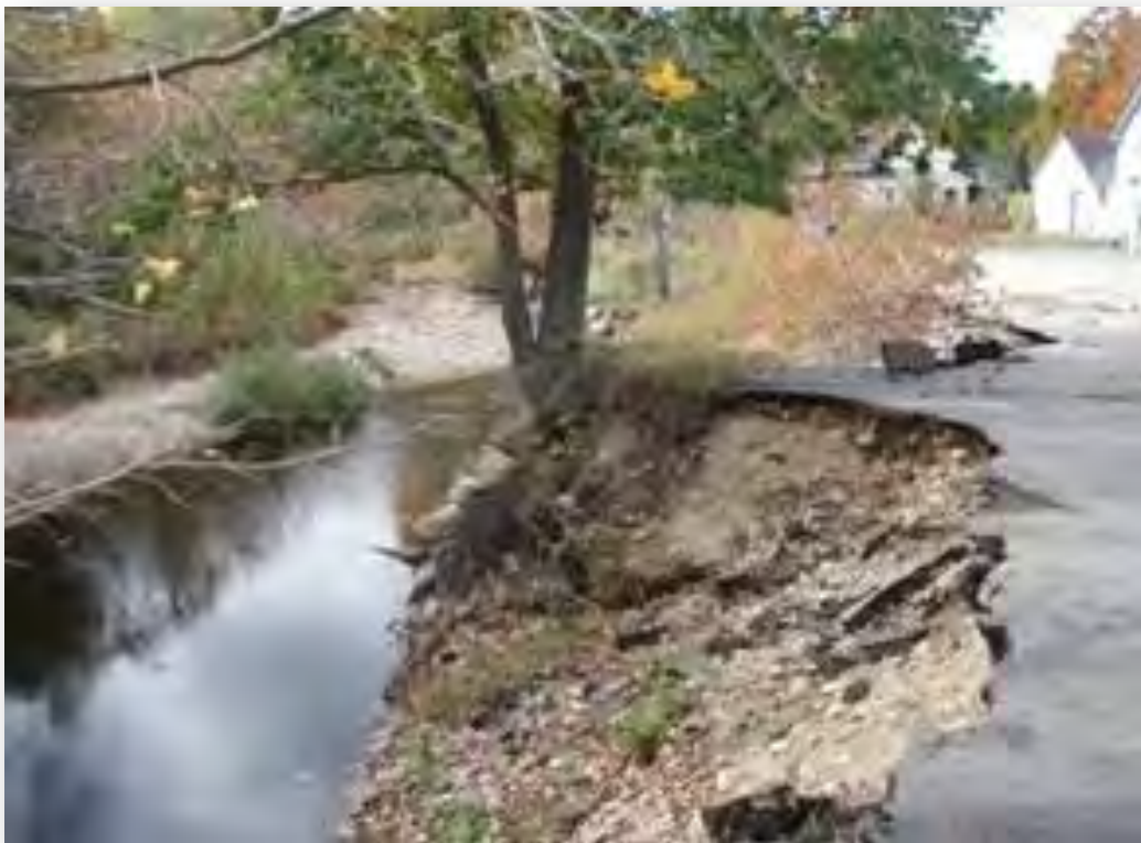
Eroded streambank from flooding at St. Peter Church
