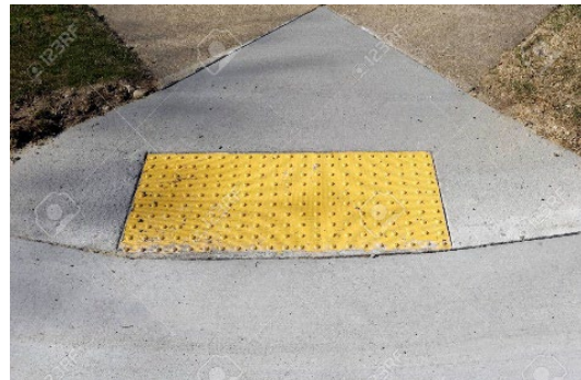
Figure 1: Ground Surface Indicators are the bumpy surfaces used on ramps to transition from the sidewalk to the crosswalk.
