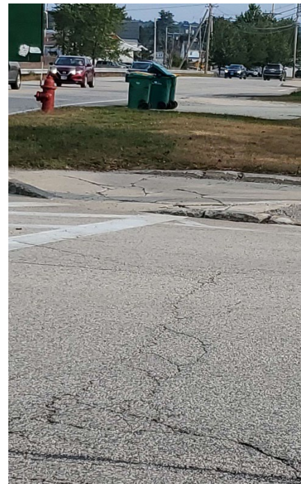
Figure 2: Crumbling sidewalk and street crossing on Summer Street
