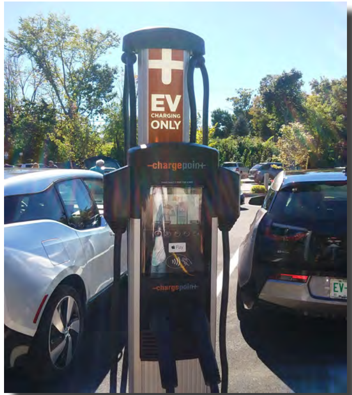
Durham EV Charging Station at Pettee Brook Source: SRPC
