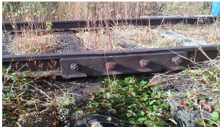
Fig. 3: Vegetation growth and poor tie condition
